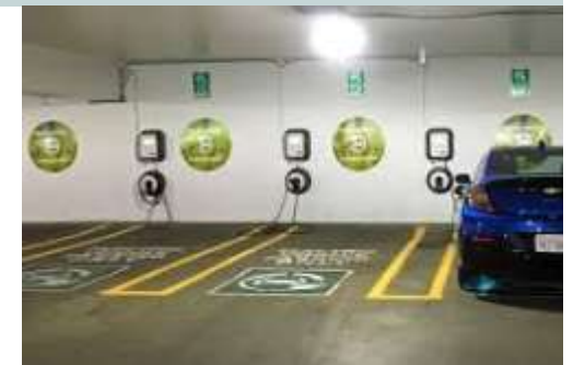
Car park provision of slow chargers
